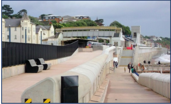
The completed sea wall as seen in July 2023, but part of the new footbridge is still seen being built.
